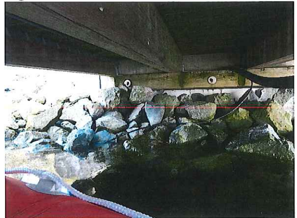
KLWI901_A_2019H_TELEFONKABEL F-1 ZERRISSEN
